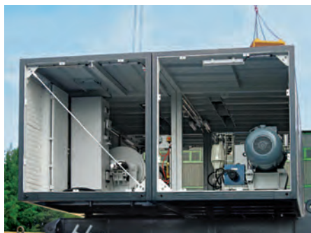
↑ Hoist gear box
