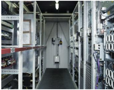
↑ Open switch cabinets are becoming more and more widely accepted
