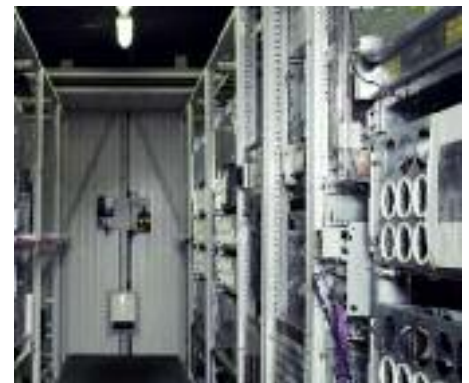
↑ Open electrical racks increasingly popular
